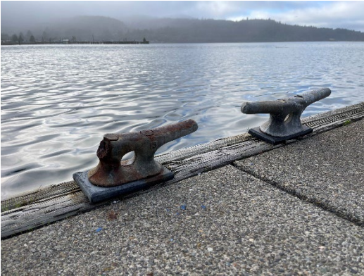
Figure 42: Broken cleat in Neah Bay along Dock A (WA EMD)
