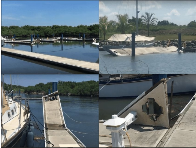
Figure 41: Dock damage in Marina Chiapas after the 2017 earthquake and tsunami. (Maria Teresa Ramirez-Herrera, 2017)
